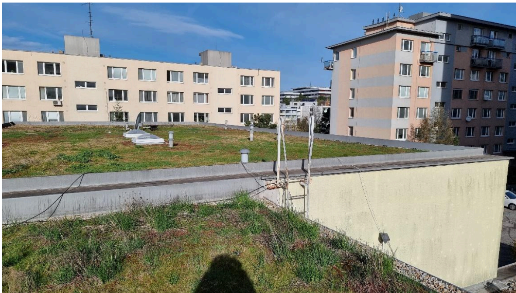
Green measure – the vegetation roof on the ARCHA senior citizens' home in Bratislava (author: Eva Pauditšová, 2023)
